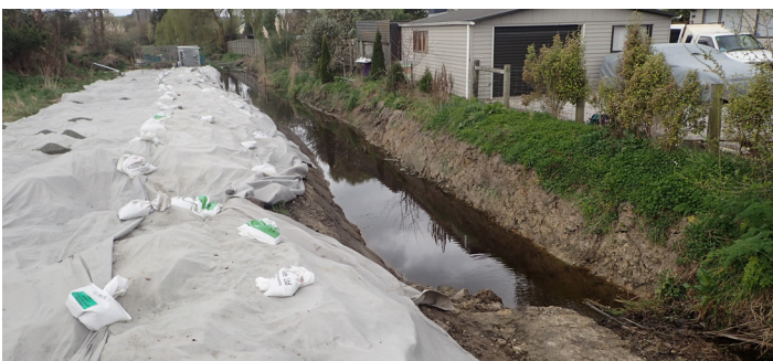
Good intentions to cover disturbed land, however no work has been done to manage sediment from the channel itself.
