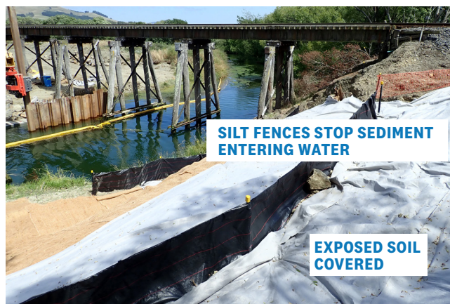
Coffer dam (yellow device in water) limits area sediment travelling further if it does reach water
