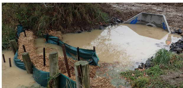
Water through this catchment has overwhelmed the sediment controls.
