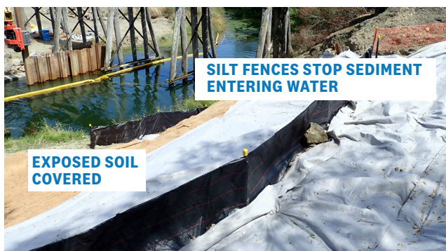
Coffer dam (yellow device in water) limits area sediment travelling further if it does reach water.
