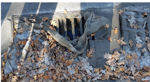
Sediment controls only work if they are regularly maintained: unfortunately filter sock has been moved and not put back in place
