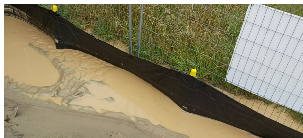
Monitoring to ensure that sediment that has been mobilised is not overwhelming the controls.
