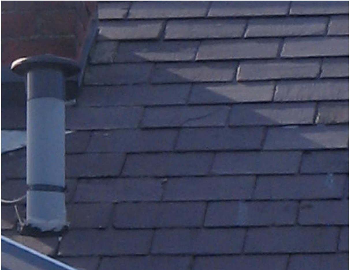
Figure 20: Slates near kitchen chimney
