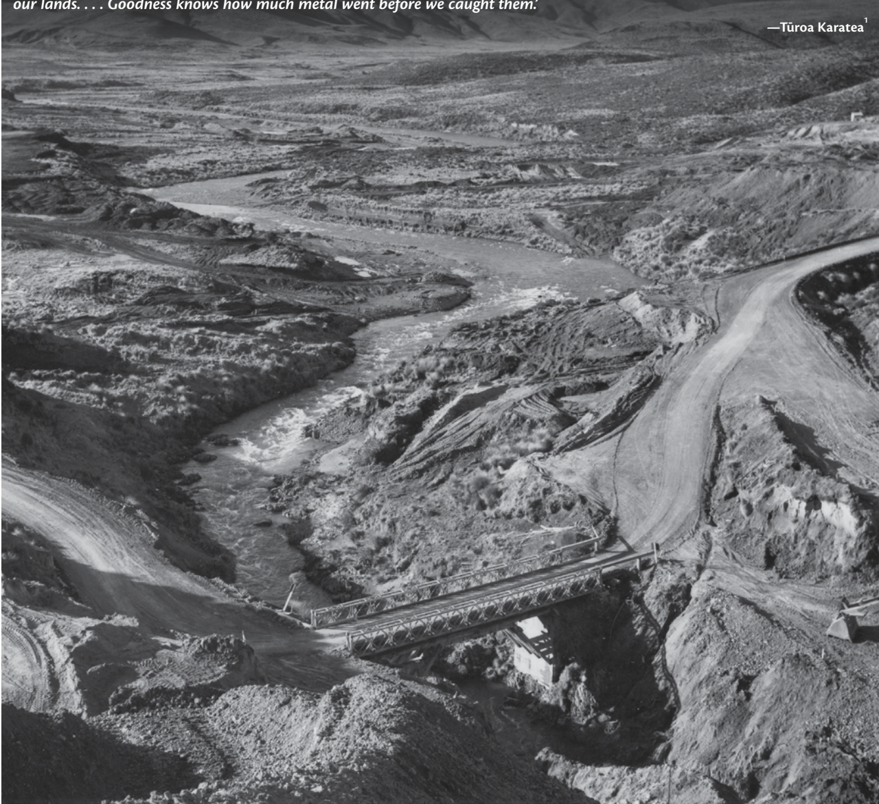
One of many access roads built for the Tongariro power development between 1964 and 1984. This one, seen in 1970, crosses the Moawhango River.
