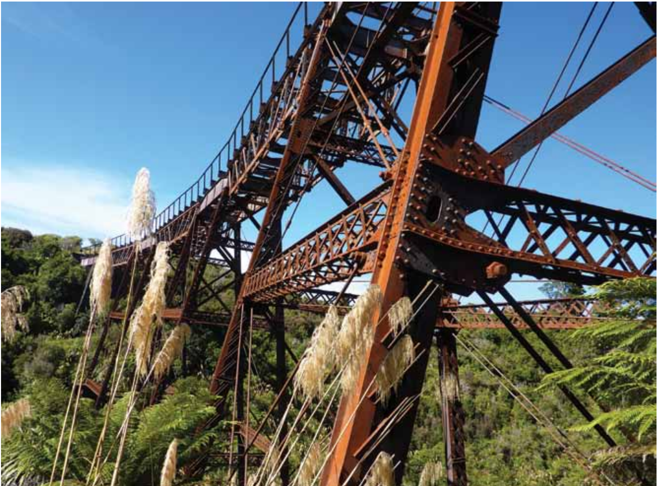
The Taonui Viaduct on the North Island main trunk railway near Horopito. Land between Horopito and Ōhakune was taken for the railway under public works legislation.
