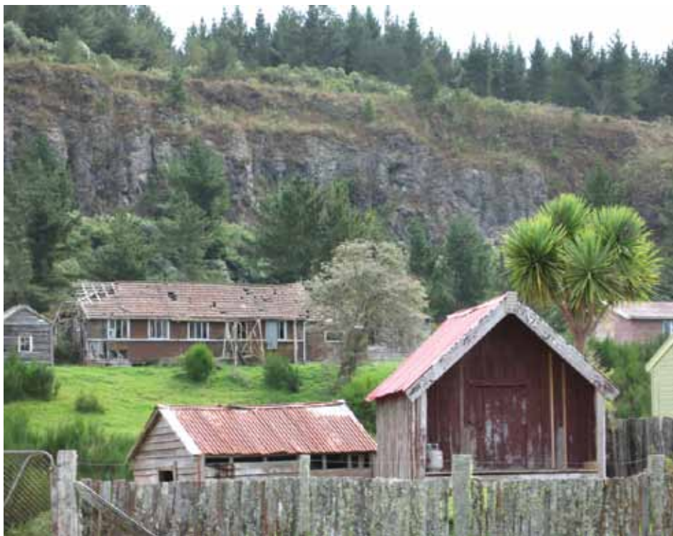
Abandoned Ministry of Works buildings. Since the workers departed, these dilapidated buildings have just been left and have deteriorated.
