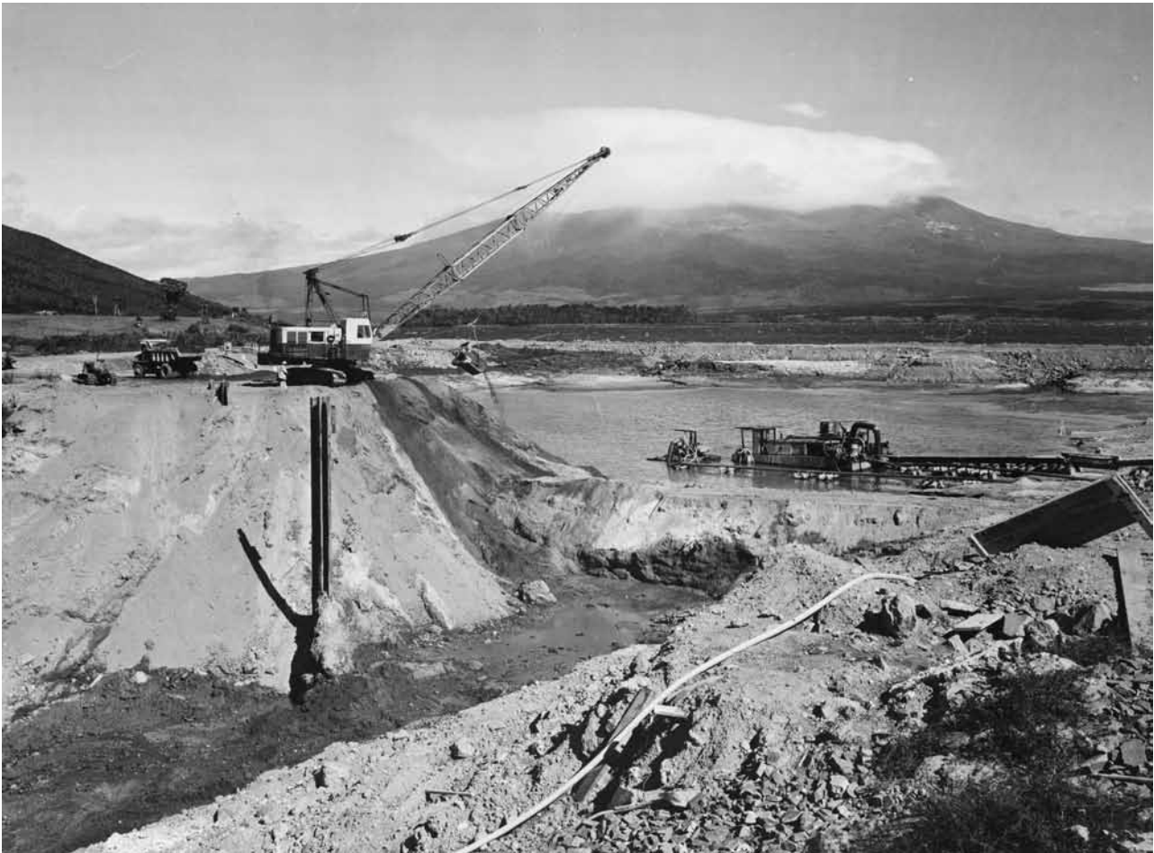
A dragline removes the final spoil from in front of the portal at Lake Rotoaira. The Tongariro power development significantly altered water flows in the lake and the Poutū Stream, thus affecting the environment.
